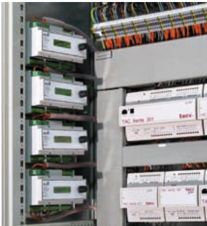
The four Fan Optimisers (left) and the TAC DDC controllers.
